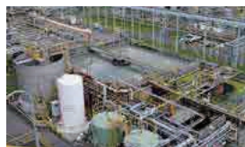
Activated sludge treatment facility
