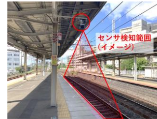
Platform safety screens
