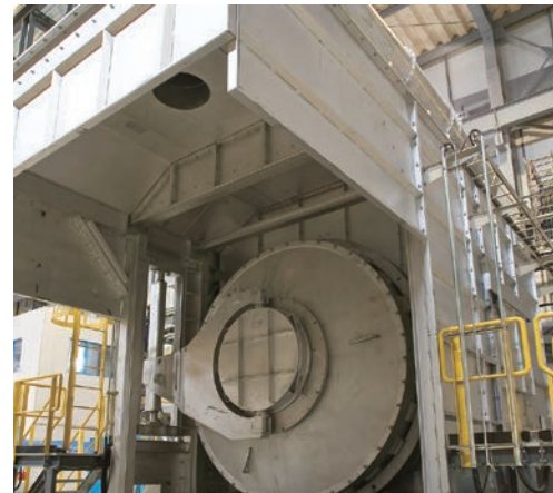
Daiseki-MCR Co., Ltd.'s rotary gas melting furnace.
