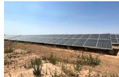
Solar power plant in Sabha, Mafraq (Jordan)
