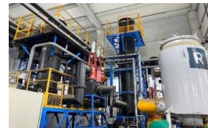
Biomass gasification power plant in Goynuk, Bolu Province in northwestern Turkey
