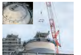
Example of reducing work in high locations by using high-precision 3D measurement data generated with drones
