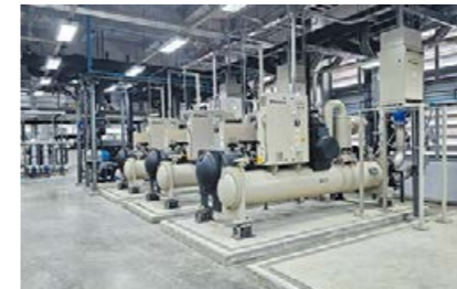
Thailand THAI OTSUKA (air conditioning work)
