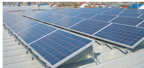
Solar power generation equipment
