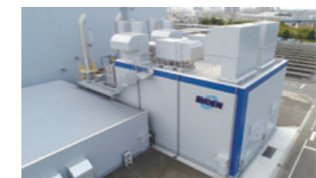
Cogeneration system (Ogaki Central Plant)
