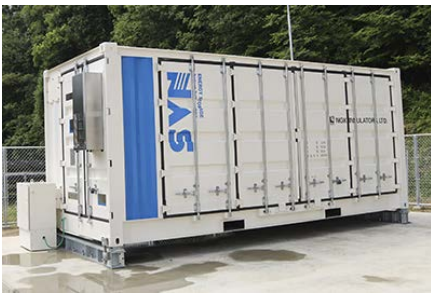
ENA ELECTRIC POWER, Yoshida Power Plant
