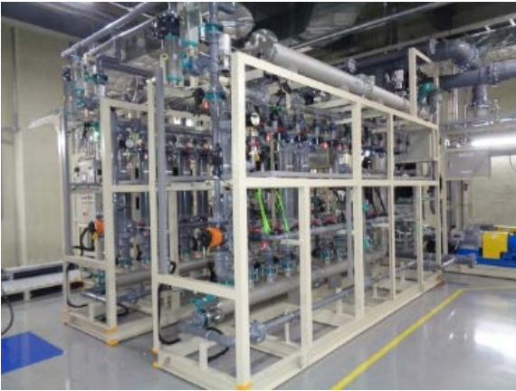
Water reclamation system in operation at NCDK Fujiyoshida Plant
