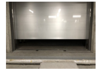
Ricoh Technology Center Watertight shutter (B1F)
