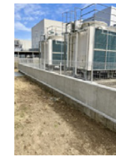
Ricoh Industry Tohoku Office Emergency generator waterproof barrier
