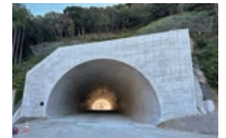
Construction of Susami Kushimoto Road-Arita Tunnel and other projects (Wakayama Prefecture) Customer: Ministry of Land, Infrastructure, Transport and Tourism
