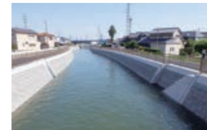
Shin Nobi (Stage II) Agricultural land disaster prevention project Shinkizu Irrigation Canal Repair work in Komaki Higashi-Tanaka construction area (No. 2) (Aichi Prefecture) Customer: Ministry of Agriculture, Forestry and Fisheries
