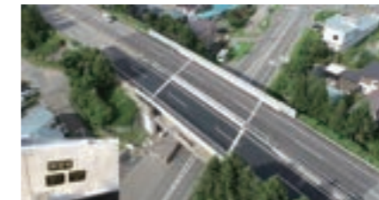
Repair work of floor slab of Jimba Bridge, Tohoku Expressway (Akita Prefecture) Customer: East Nippon Expressway Company Limited
