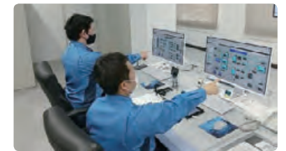
Renewed monitoring and control equipment
