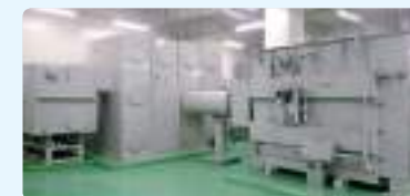
Renewed extra-high power receiving and transforming equipment
