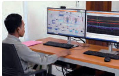
Monitoring and control of sewage treatment plants by local operators
