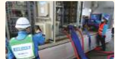
Our technical staff (foreground) setting up an in-vehicle ceramic membrane filtration system with Imabari City officials
