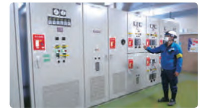
Renewed electrical equipment
