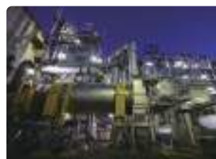
Sludge Fuel Conversion Plant at the Kosei Sewage Treatment Center, which has successfully implemented unmanned nighttime operation
