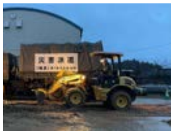
Clearing the elementary school grounds at the evacuation center to make it easier to walk.
