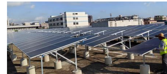
Dongguan Factory Solar Power Generation
