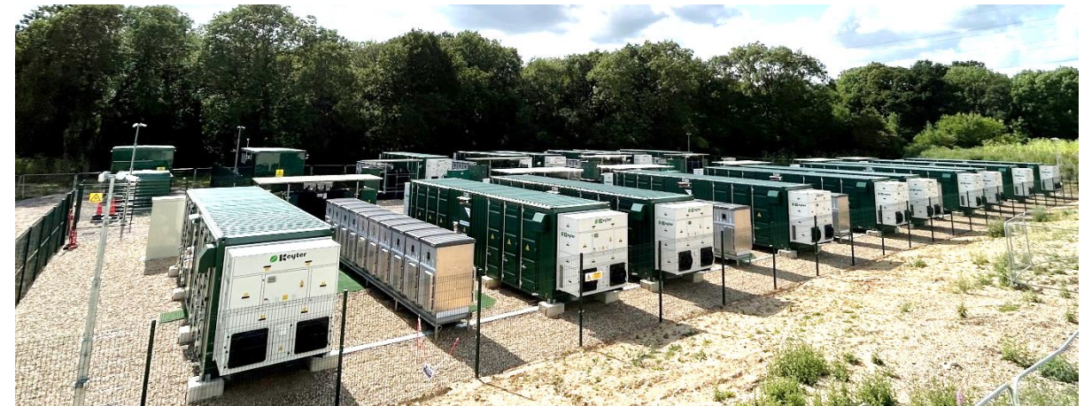
"Project Lion" Power storage project for the grid in the UK
