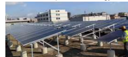
Dongguan Factory Solar Power Generation
