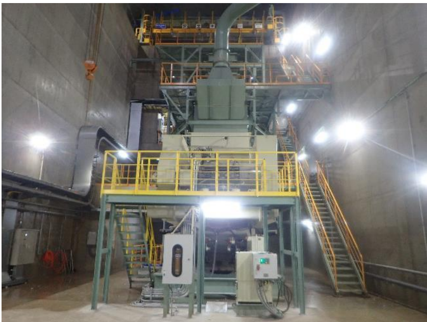
Crusher at the third vertical shaft
