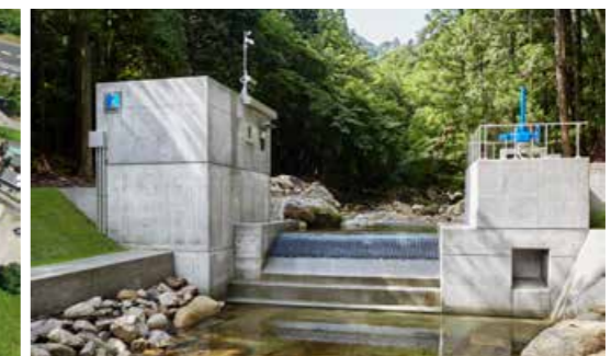
Kamogawa Small Hydroelectric Plant
