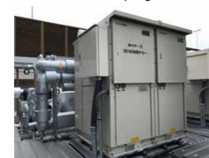
Heat pump that use river water
