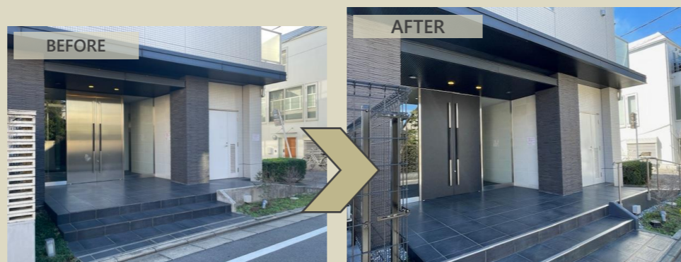
Changed the color of the entrance door and added handrails to the slope to prevent falls
