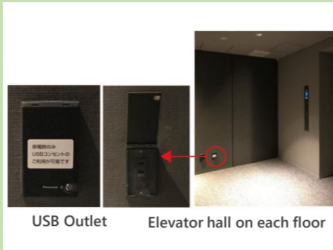
Emergency power supply by storage batteries
