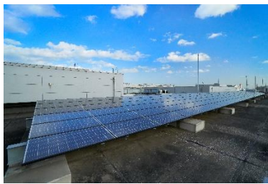
Utilizing natural energy
