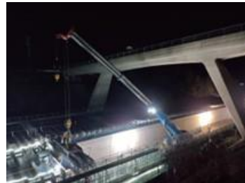
Joshin-Etsu Expressway Yomogidaira construction project JV of Fujita Corporation and MMB East Nippon Expressway Company Limited
