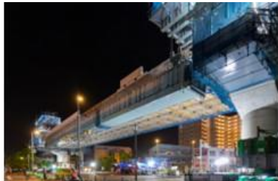
Sasebo Viaduct widening construction on the Sasebo Road JV of MMB, The Takigami Steel Construction, and Fuji P.S West Nippon Expressway Company Limited
