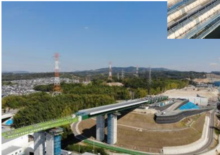
Constructino work of Shin-Meishin Expressway the First Jojo viaduct West Nippon Expressway Company Limited
