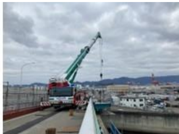
Kobe Airport Access Bridge superstructure (widening) manufacture and erection JV of MMB and YORIGAMI MARITIME CONSTRUCTION Kobe City
