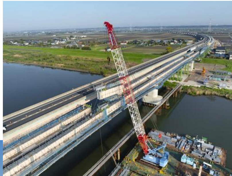
Construction work of the Superstructure of R3 Kenoudou Tone River Bridge Kanto Regional Development Bureau
