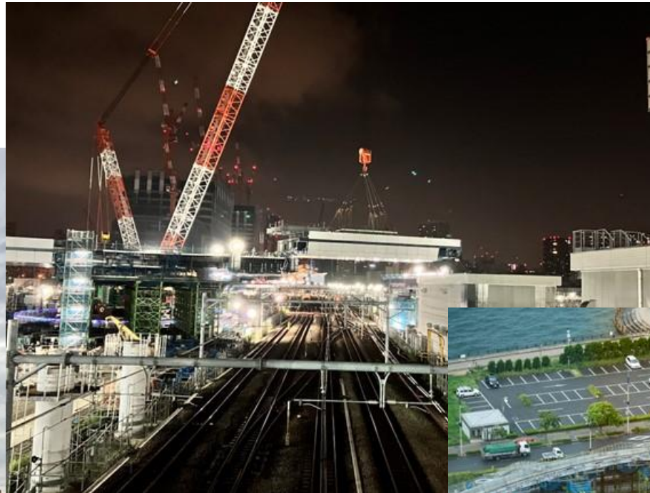
New construction of crossing section of Kanjo 4 Expressway within Shinagawa Station building, etc. Kajima Corporation
