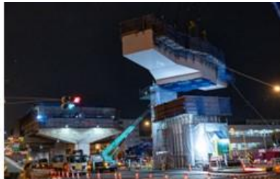
Kire-Uriwari Bridge large-scale renovation project Industry-spanning JV of TAISEI, Fuji P.S. and MMB Hanshin Expressway Company Limited
