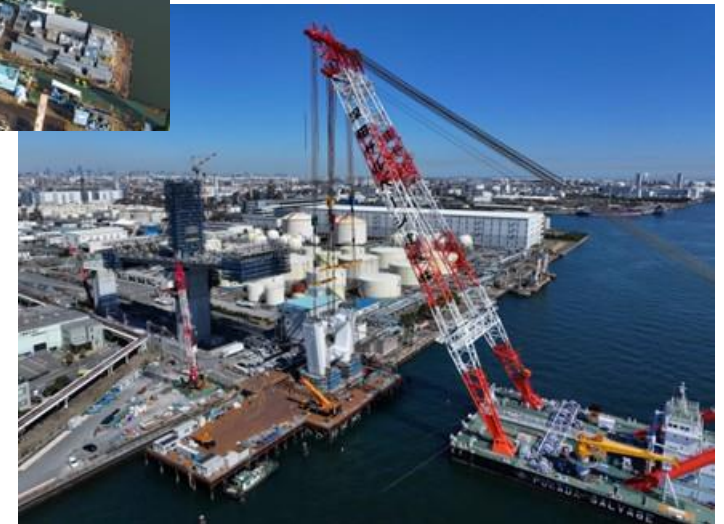
Construction work of the superstructure of the main bridge on Kawasaki harborroad Higashi Ogishima Mizue-cho line, 1st Kanto Regional Development Bureau
