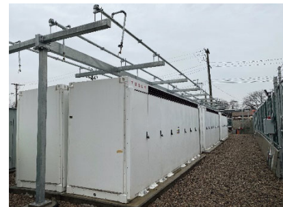
System battery facility developed with Summit Ridge Energy, LLC (New York, US)
