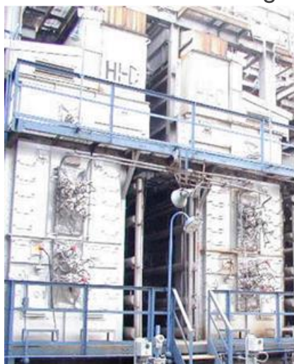
Naphtha cracking furnace where demonstration experiment was conducted
