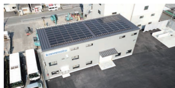
Solar Power Generation System Installed on the Roof of the Kyoto Branch Office
