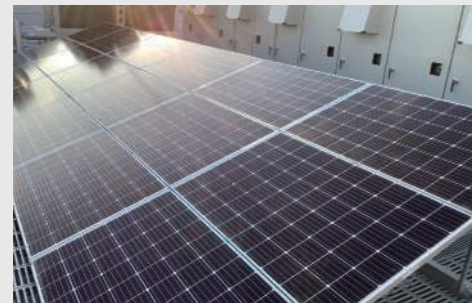
Solar panels installed at our headquarters
