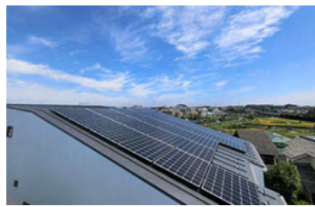
Solar power generation system
