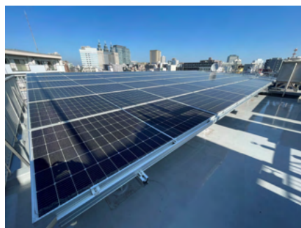
T's eco Kawasaki Solar Panels
