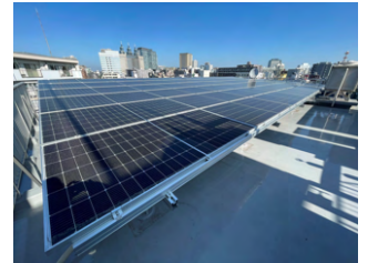
Solar panels installed on the rooftop
